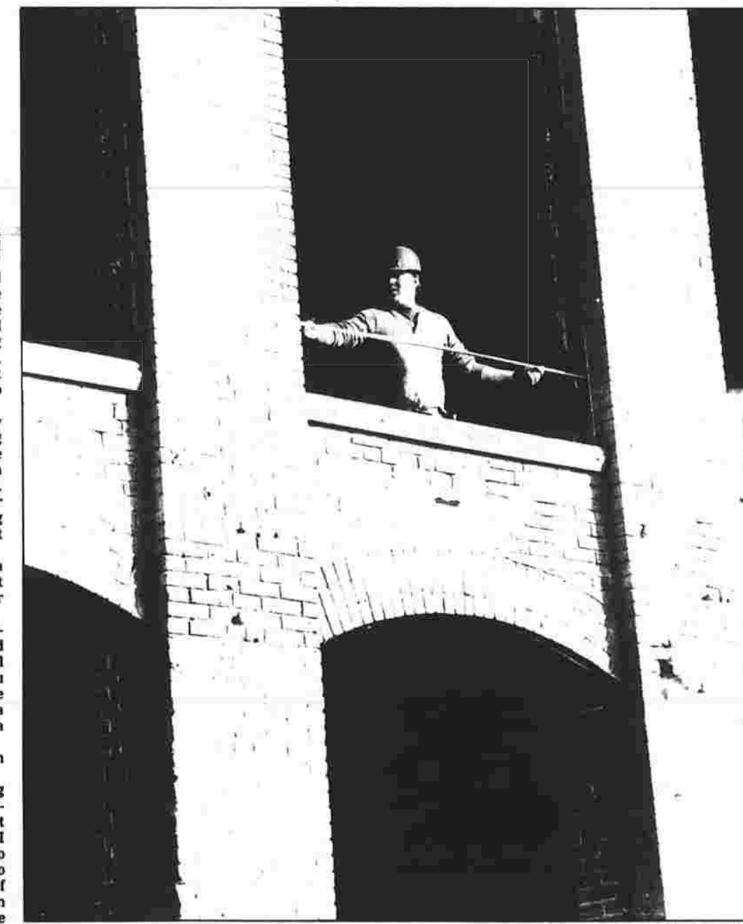
LOOKING AHEAD — Tony Bonito, 26, takes a measurement for installing a new window in the former Cheney Brothers Yarn Mill at 210 Pine St. today. The conversion of the mill will be into 103 residences and eight stores should be complete in nine to 11 months, the developer, Brophy Ahern of West Haven said today. Brophy Ahern received building permits for the mill Tuesday. Story on page 3.
